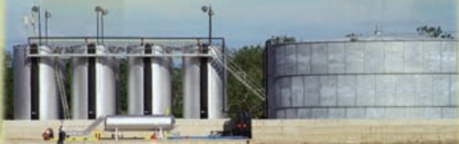
Separation unit and storage tanks at Iguana Creek
